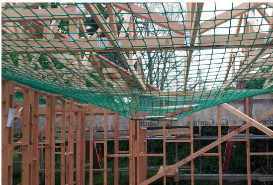
Figure 15: Debris must be removed from safety nets.
